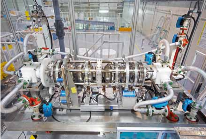
Figure 2.2 The EP facility established at KEK-STF.
